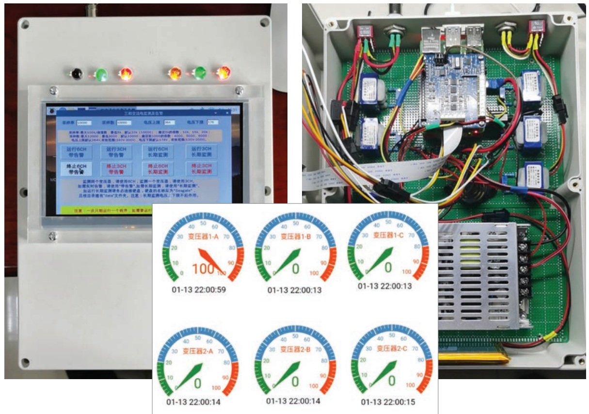
The completed system includes a Raspberry Pi 4, the MCC 118 DAQ HAT, six transformers for the 220 V signals and a power supply. The external view shows the alarm LEDs and a screen with real time data.
